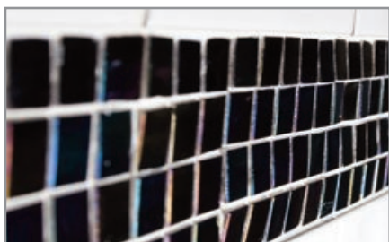
An unacceptable finish when bedding out
